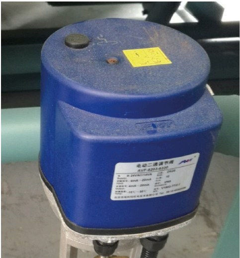
Figure 29: Actuator for drain control valve
