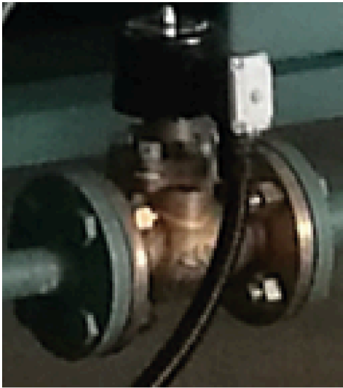
Figure 28: Steam drain solenoid valve
