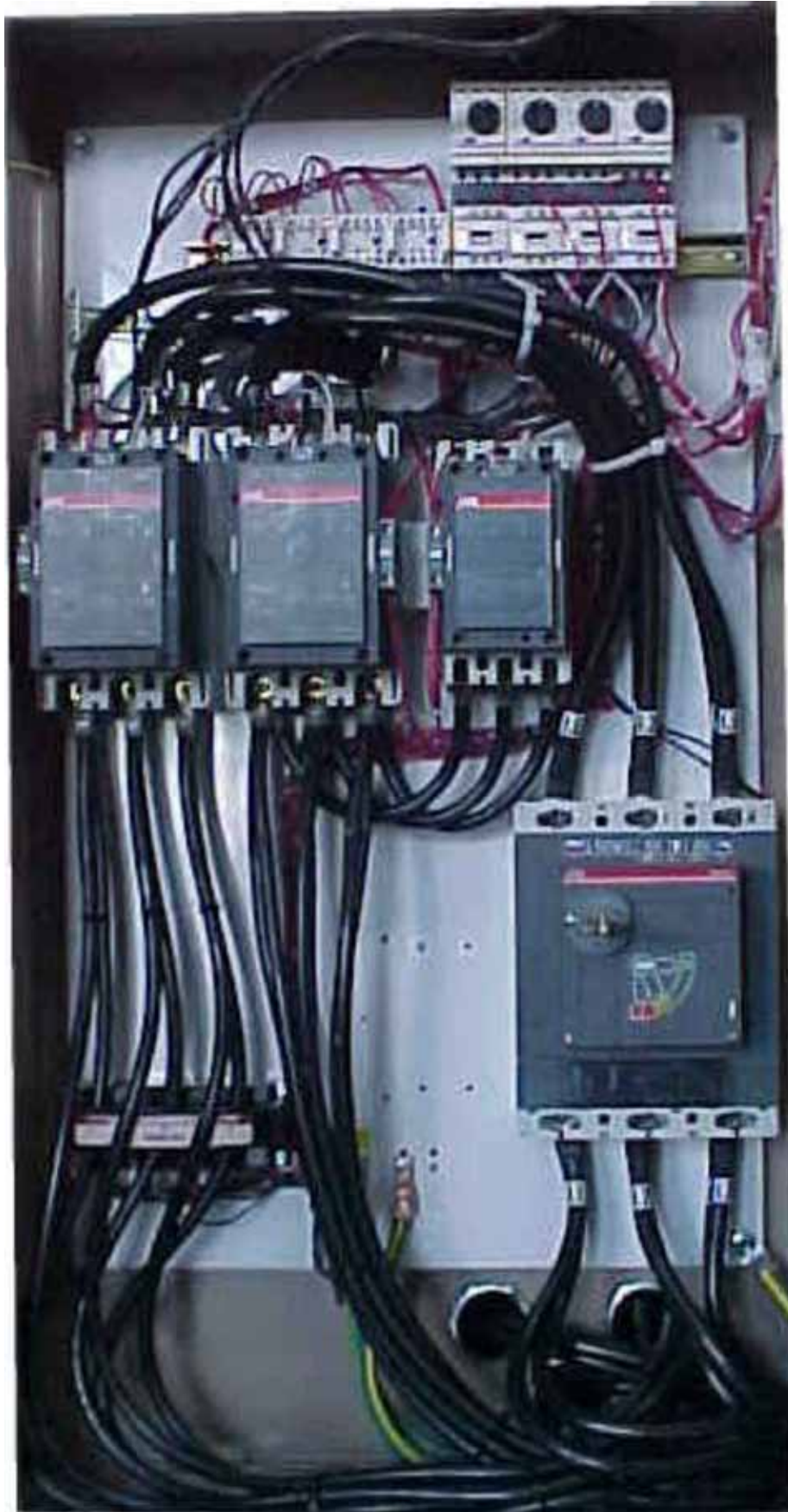
FIG. 12 – WYE DELTA POWER PANEL
