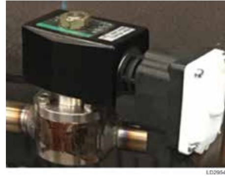
FIGURE 20 - SOLENOID VALVE FOR PURGE AND BLOW PUMP
