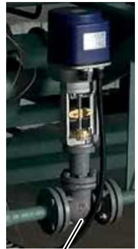
Steam drain control valve
