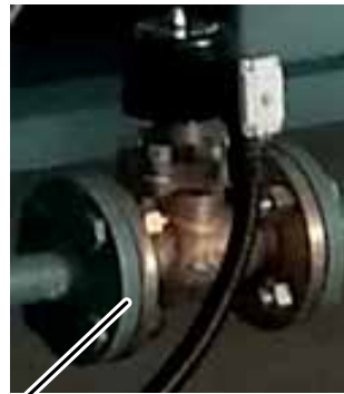
Steam drain solenoid valve
