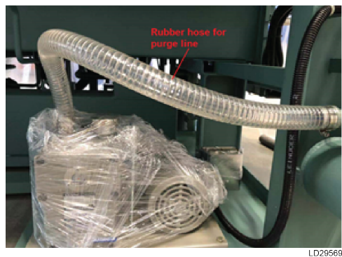
Figure 38: Rubber hose for purge line
