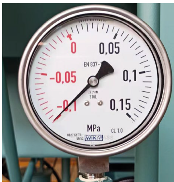
Figure 37: Compound gauge for purge line
