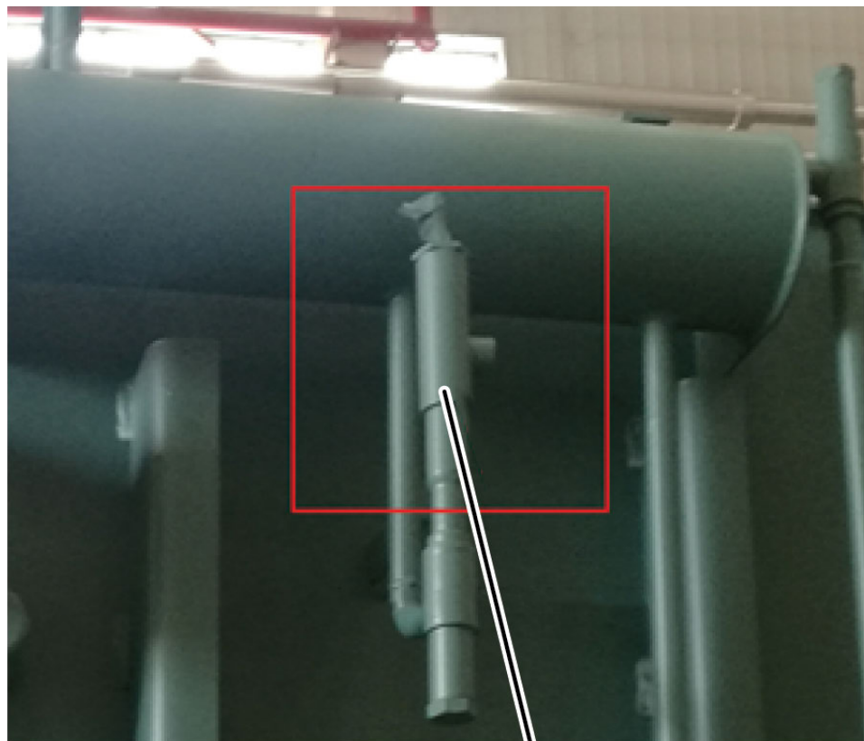
Pressure Release Valve
